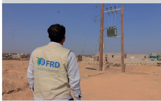
FRD implements electrical supply projects.
