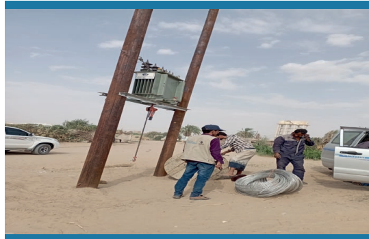
ACTED implements electricity supply projects.
